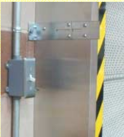
(Above) Metal sheeting covers the side of the guide tracks to provide a secure seal.
